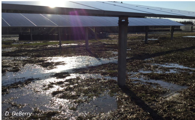
Figure 2-2: Example of surface water ponding on poorly-drained and compacted soil at a solar facility during construction.
